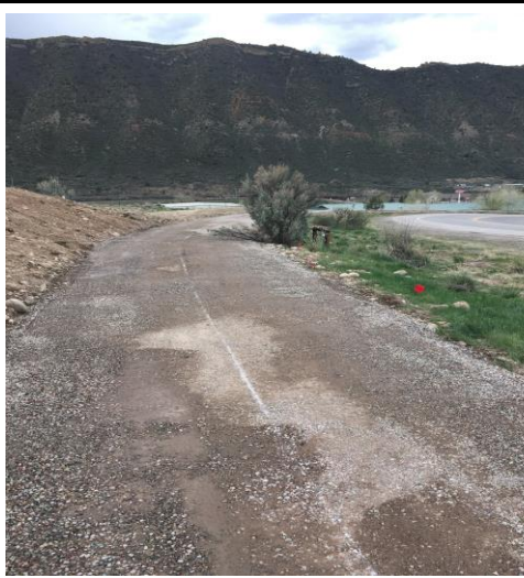
Town of New Castle Public Works is busy building a trail from the Shibui Apartments to the City Market Plaza.
