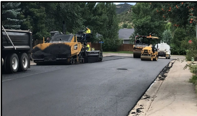
The 2023 street paving projects were in full swing in August. Crews milled and paved on Current Dr, Penny Royal, E Capital, Rio Grande, Oak Ct, Mesquite Ct, Lupine Dr, Dragon Root, and Mallow Ct.
