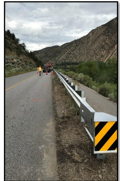
The guard rails along 335 Road have been replaced thanks to a grant from the Colorado Department of Transportation.
