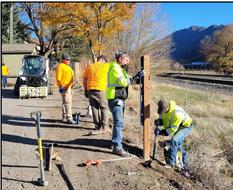
New Castle Public Works begin installing the new back-alley fence, funded by a grant from FMLD.
