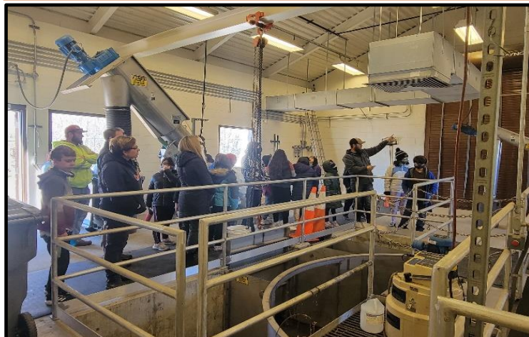
Elk Creek Elementary students tour the wastewater treatment plant
