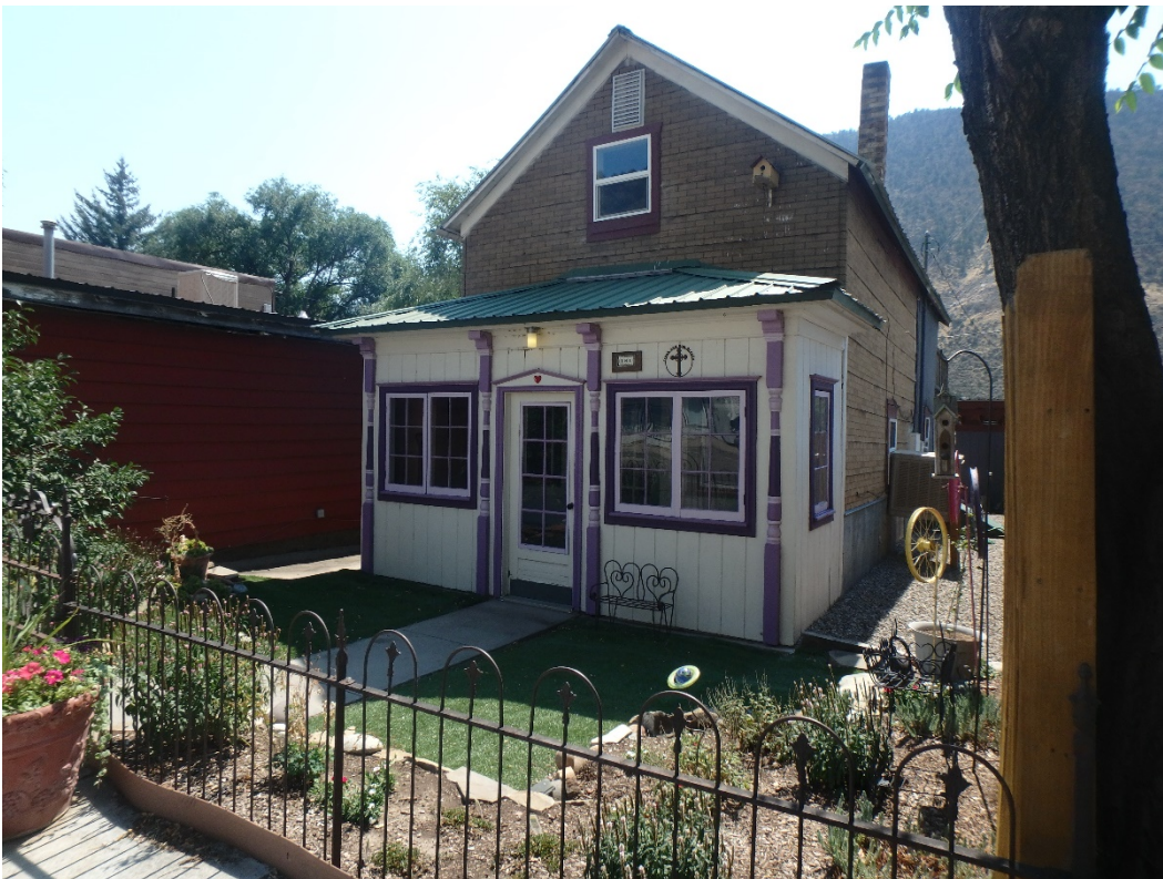
Photo Number: 5GF.2370_2 Description: Looking at the primary (north) and west elevations of the residence. Note the weatherboard, asphalt, and corrugated metal siding transitions. Date: 9/6/2022 View: Southeast
