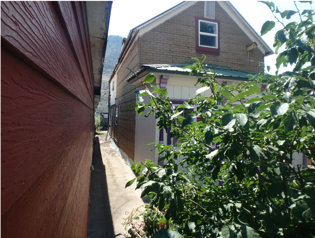
Photo Number: 5GF.2370_3 Description: Looking at the east and primary (north) elevations of the building. Date: 9/6/2022 View: Southwest
