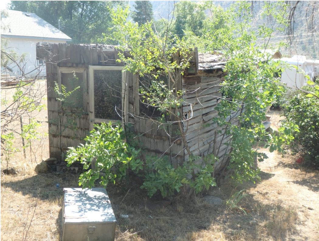
Photo Number: 5GF.5927_1 Description: Looking at the primary (north) and west elevations of the building. Note the wood shingle and horizontal weatherboard siding. Date: 9/6/2022 View: Southeast
