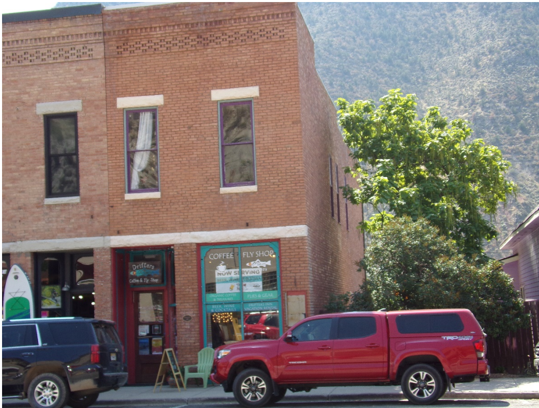
Photo Number: 5GF.2379_1 Description: Looking at the primary (north) and west elevations of the building. Note the decorative brickwork below the cornice. Date: 9/6/2022 View: Southeast
