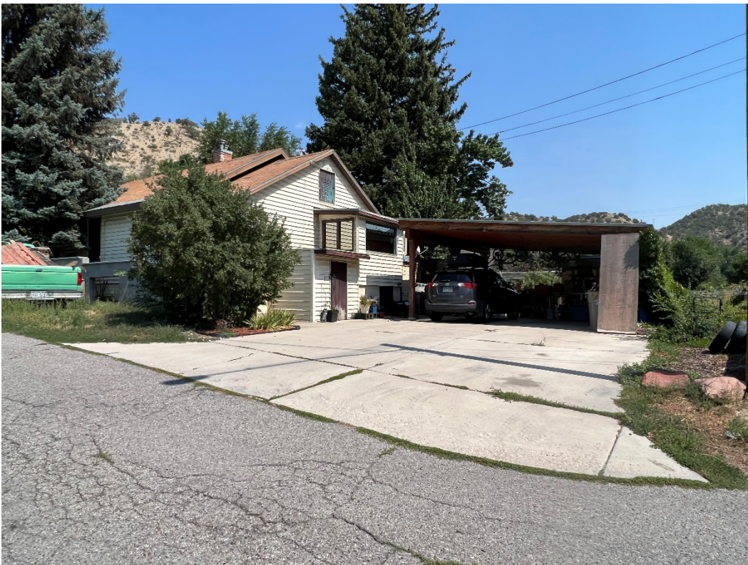
Photo Number: 5GF.5933_4 Description: Looking at the west elevation and south elevation of the building. Date: 9/6/2022 View: Northeast
