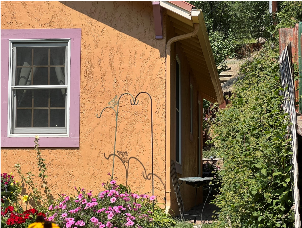
Photo Number: 5GF.5937_4 Description: Looking at the east elevation of the building. The building's proximity to the wall on the right makes it difficult to observe the entire elevation. Date: 9/6/2022 View: Northwest
