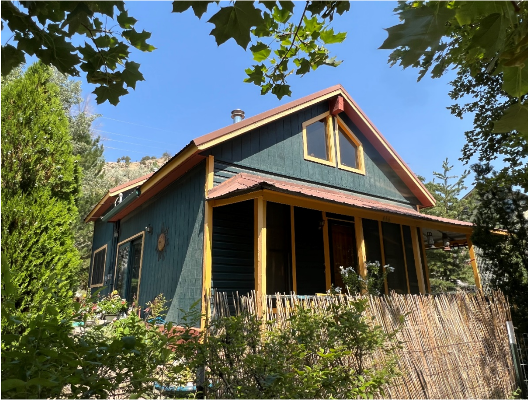
Photo Number: 5GF.5938_1 Description: Looking at the west and primary (south) elevation of the building. Date: 9/6/2022 View: Northeast
