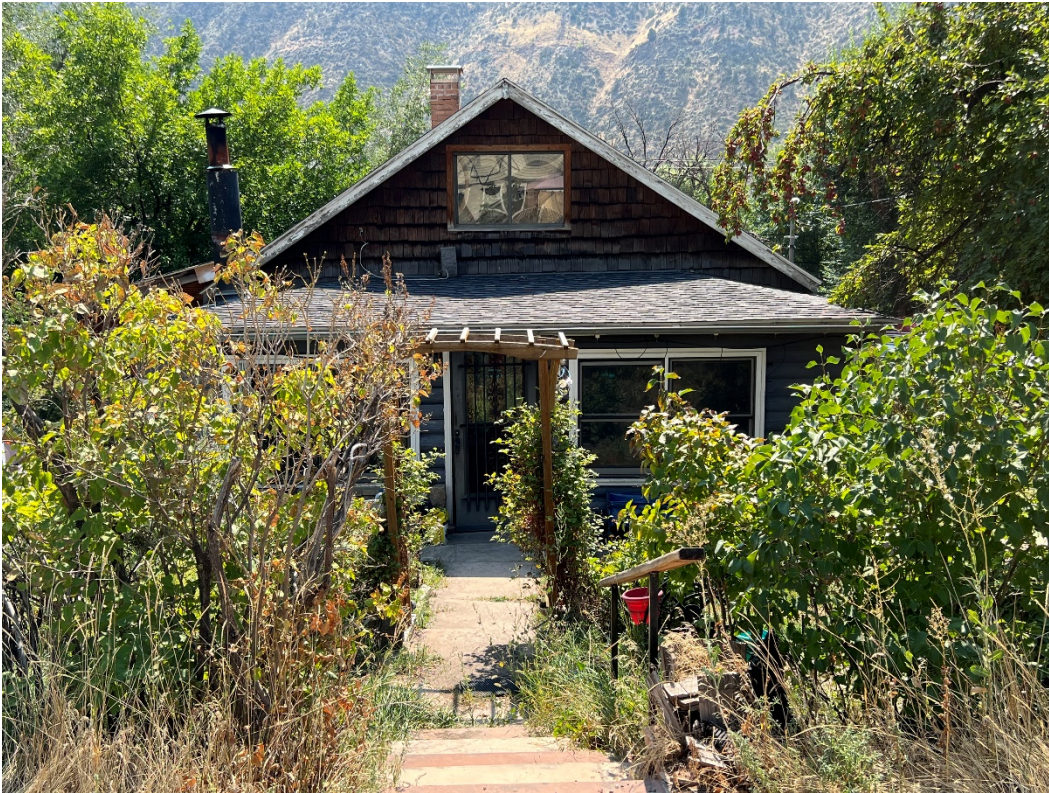
Photo Number: 5GF.5939_1 Description: Looking at the primary (north) elevation of the building. Note the wood shingles under the gable end. Date: 9/6/2022 View: South
