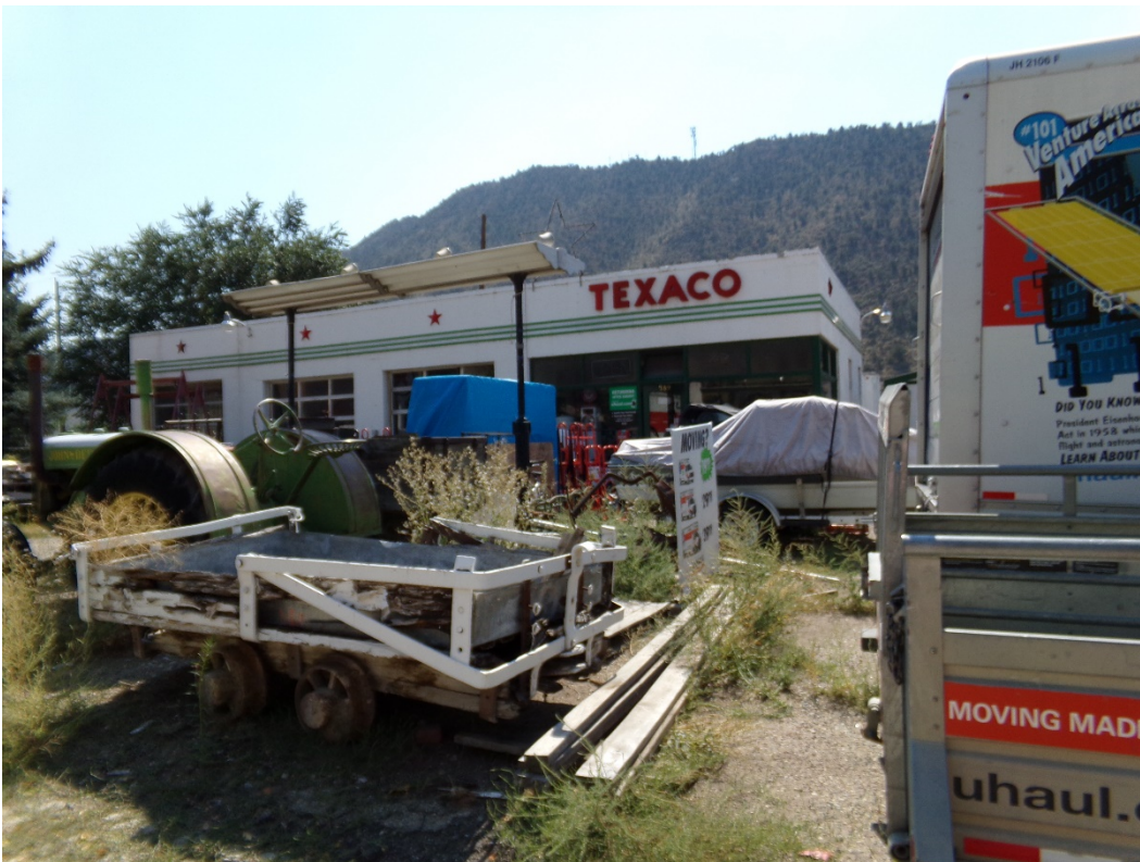
Photo Number: 5GF.5903_2 Description: Looking at the primary (north) and west elevations of the building. Note the fuel island in the foreground. Date: 9/6/2022 View: Southeast
