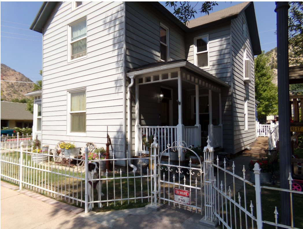
Photo Number: 5GF.5900_2 Description: Looking at the south and primary (east) elevations of the building. Date: 9/6/2022 View: Northwest
