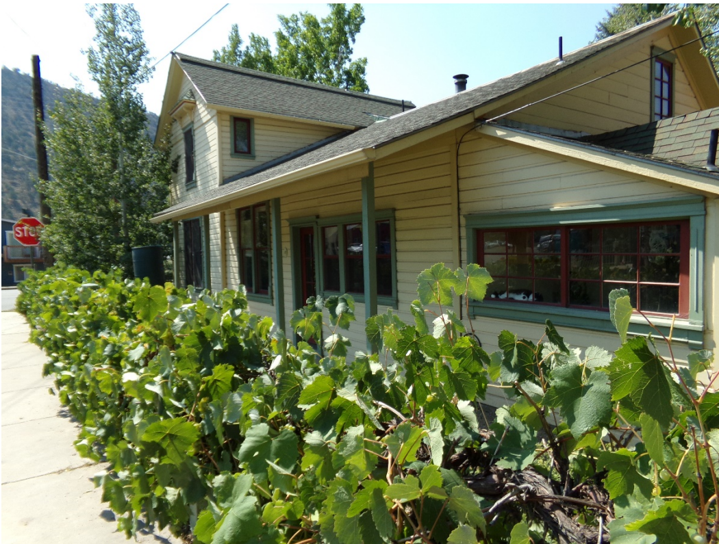
Photo Number: 5GF.5898_3 Description: Looking at the east elevation of the primary residence. Date: 9/6/2022 View: Southwest
