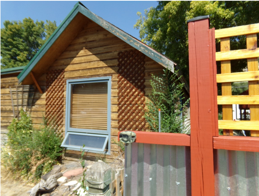
Photo Number: 5GF.5896_3 Description: Looking at the right side of the south elevation of the building. Date: 9/6/2022 View: Northwest
