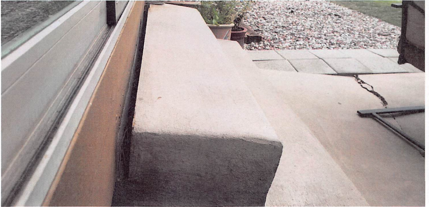
Stairs Pulling Away
