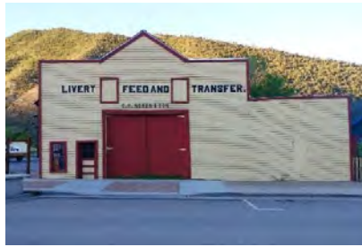
Vacant, Poor State of Repair and Storage
